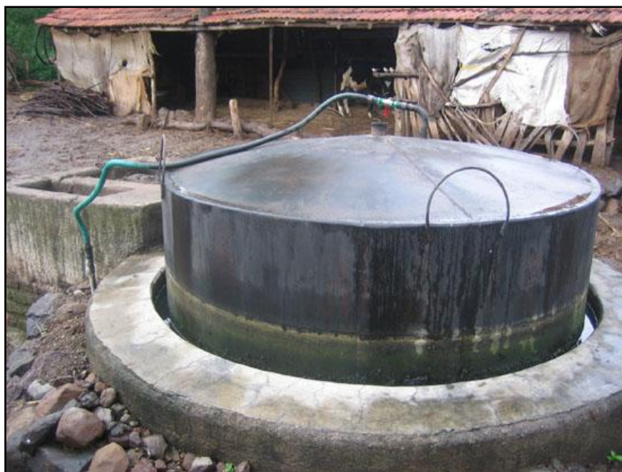
Figure 2-7. Photo of a floating drum plant in India (engINdia, 2005).
