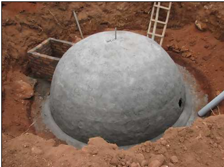
Figure 2-3. A fixed dome digester during construction. When finished most of the plant will be covered by earth (Acres Wild, 2008).
